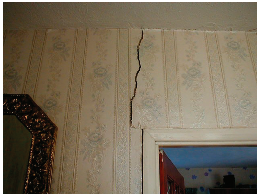
Figure 6: Internal cracking in a farmhouse in Lincolnshire caused by poplar trees 20 m away from the building
