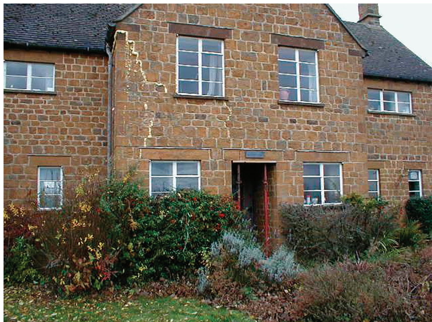
Figure 2: Severe cracking to a sandstone house in Oxfordshire caused by fruit trees growing in the garden (note the foam filling in the cracks and the jacks supporting the lintel)
