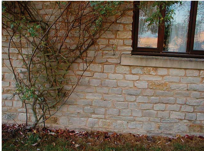
Figure 5: Cracking in a recently built house near Stratford-upon-Avon. This house is less than five years' old and the design of the foundations did not account for poplars, willows and maples growing in the garden at distances of between 10 m and 20 m from the house
